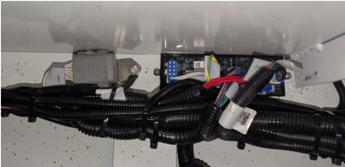
Figure 47: Harness 03034764 Connection at CEM1606
