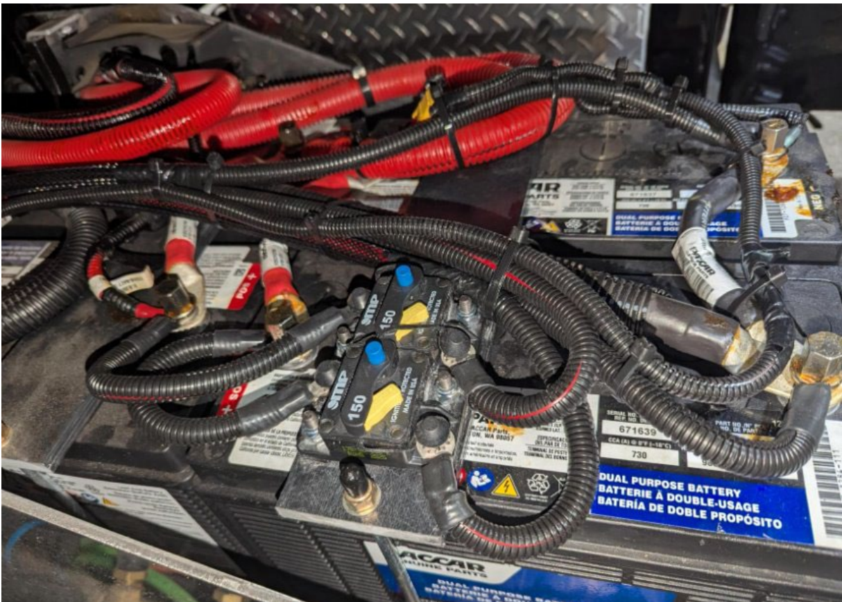
Figure 35: 150-Amp Circuit Breakers on Battery
