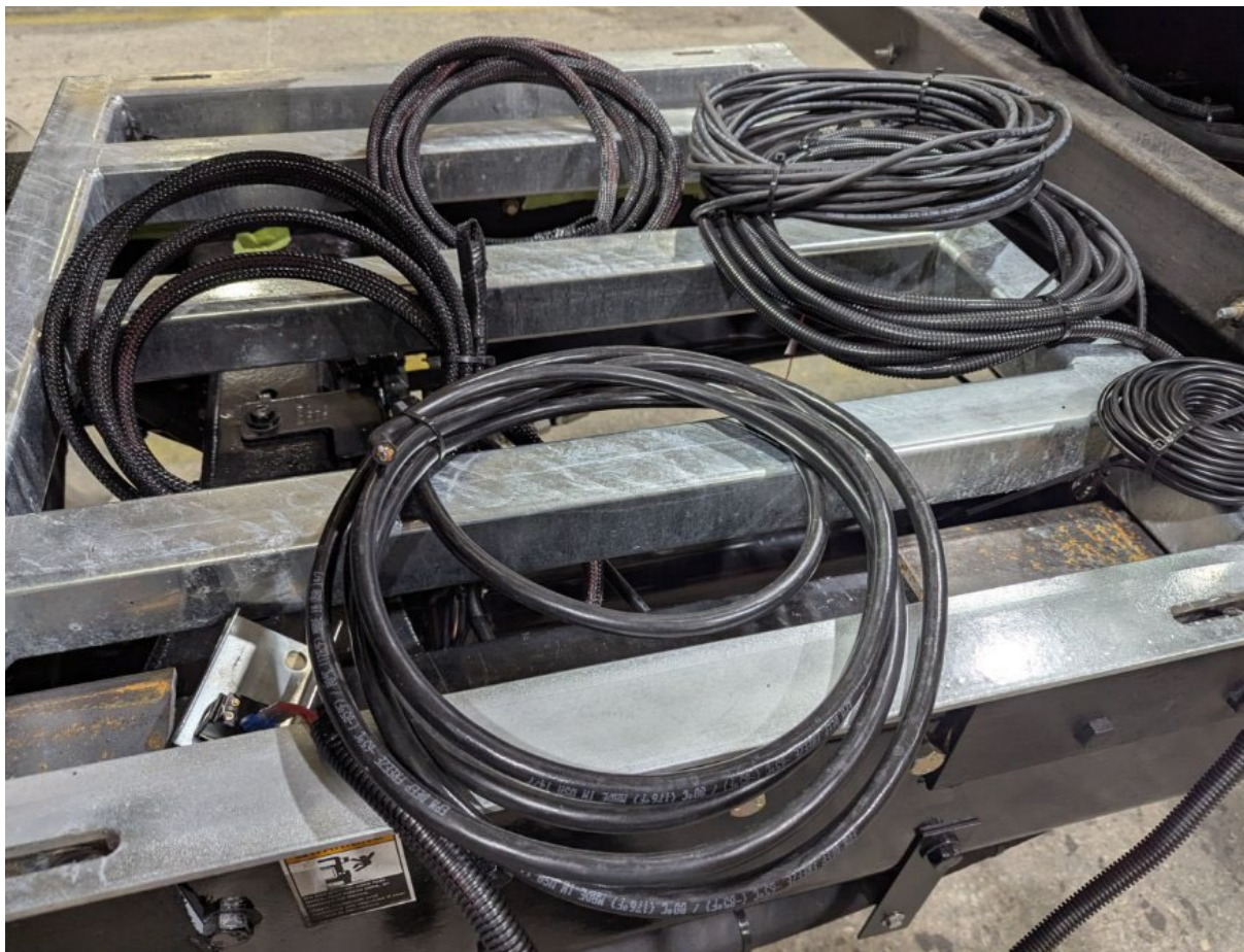
Figure 33: 4-Gauge Loomed Power/Ground Cables, Chassis Inputs Ready for Install
